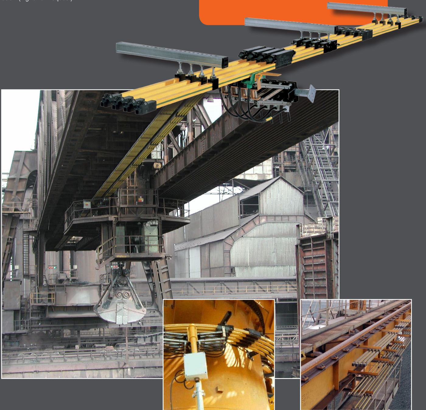
Conductor Rails on a boom stacker
